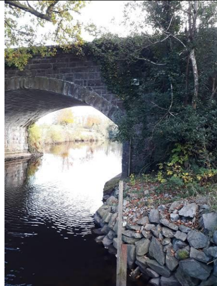
Plate 2 Aghoo Bridge, the pedestrian underpass will be connected to the right side of the bridge arch, as viewed from this image.
