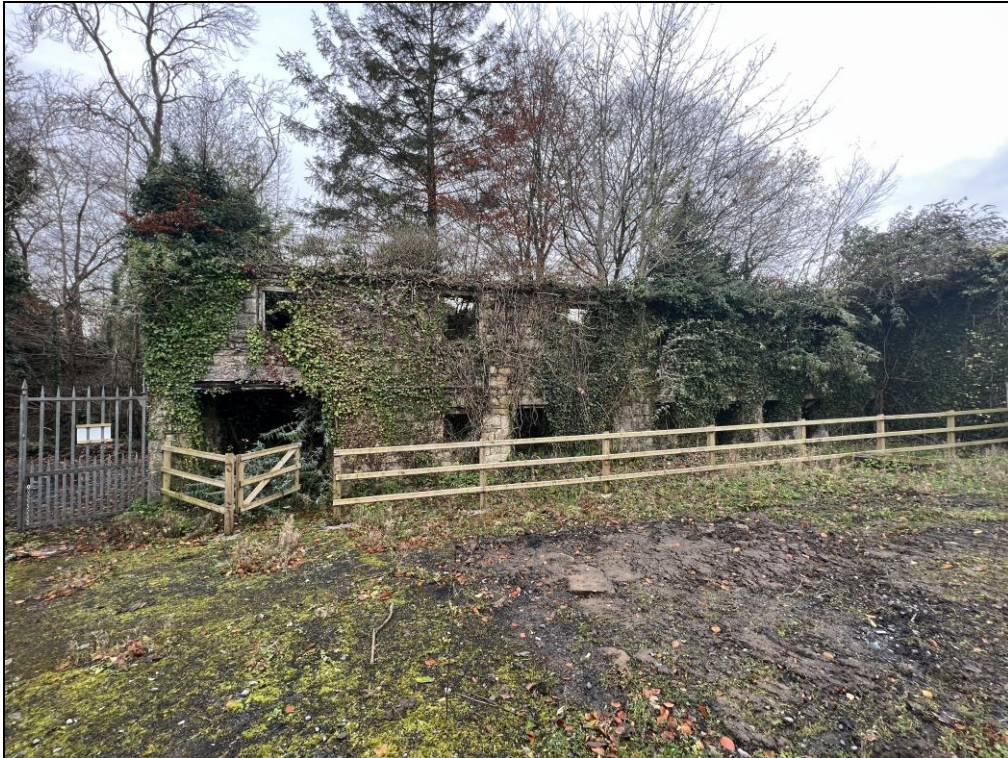
Plate 16: East facing view of the stone outbuilding to the rear of the bank, this was a former forge or smithy.
