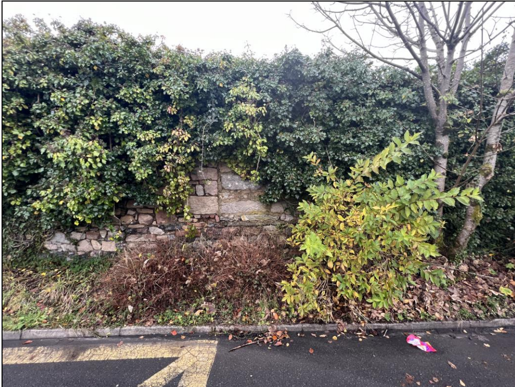
Plate 4: West facing view of the boundary wall between the carpark and the river showing trace remains of a window.
