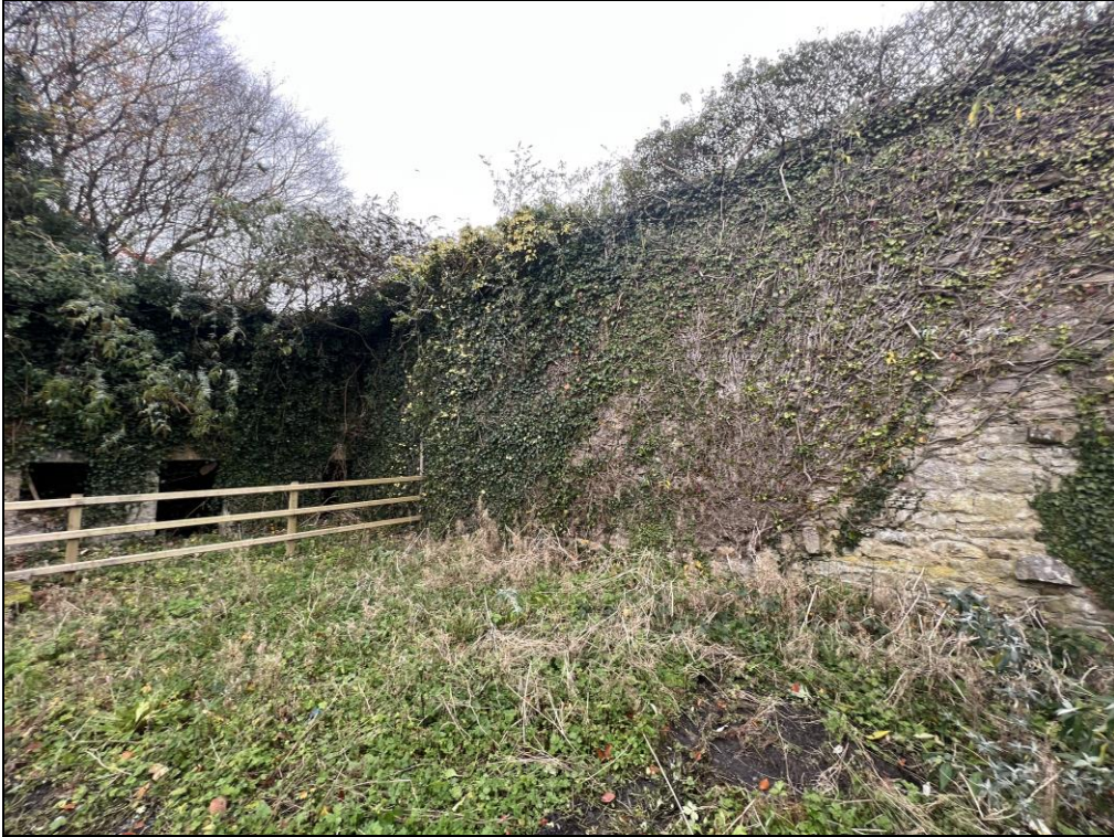
Plate 18: NW facing view of the boundary wall between the carpark and the bank site, where vehicular access is proposed to be provided through the wall.
