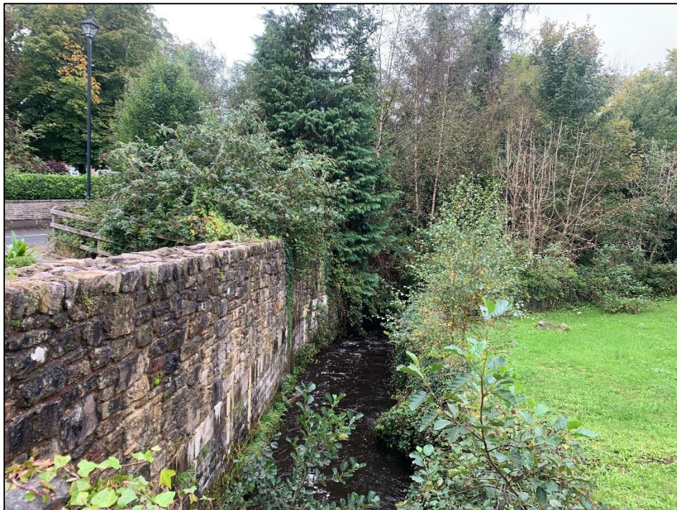
Photos 6-8: Showing the Drumshanbo River flowing through the site (Habitat Type FW2 – Lowland Rivers). This River is highly channelised with adjoining stone walls (Habitat BL1 – Stone Walls) and Habitat WN5 – Riparian Woodland (mainly Sycamore, Ash, Beech, Silver Birch, Alder and occasional Conifers)
