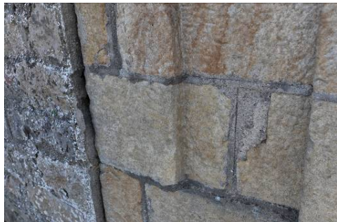
FIG. 7; OPEN JOINT BETWEEN PIER AND ADJACENT WALL, INDICATING DIFFERENTIAL MOVEMENT.
