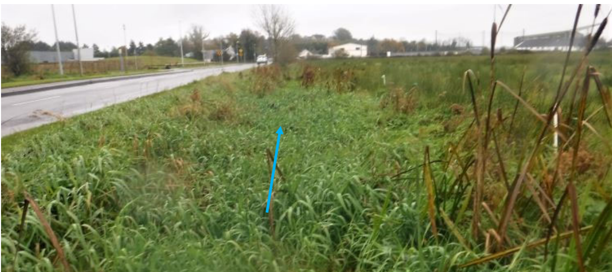
Photo 06: View South along the existing drainage ditch located along the eastern boundary.
