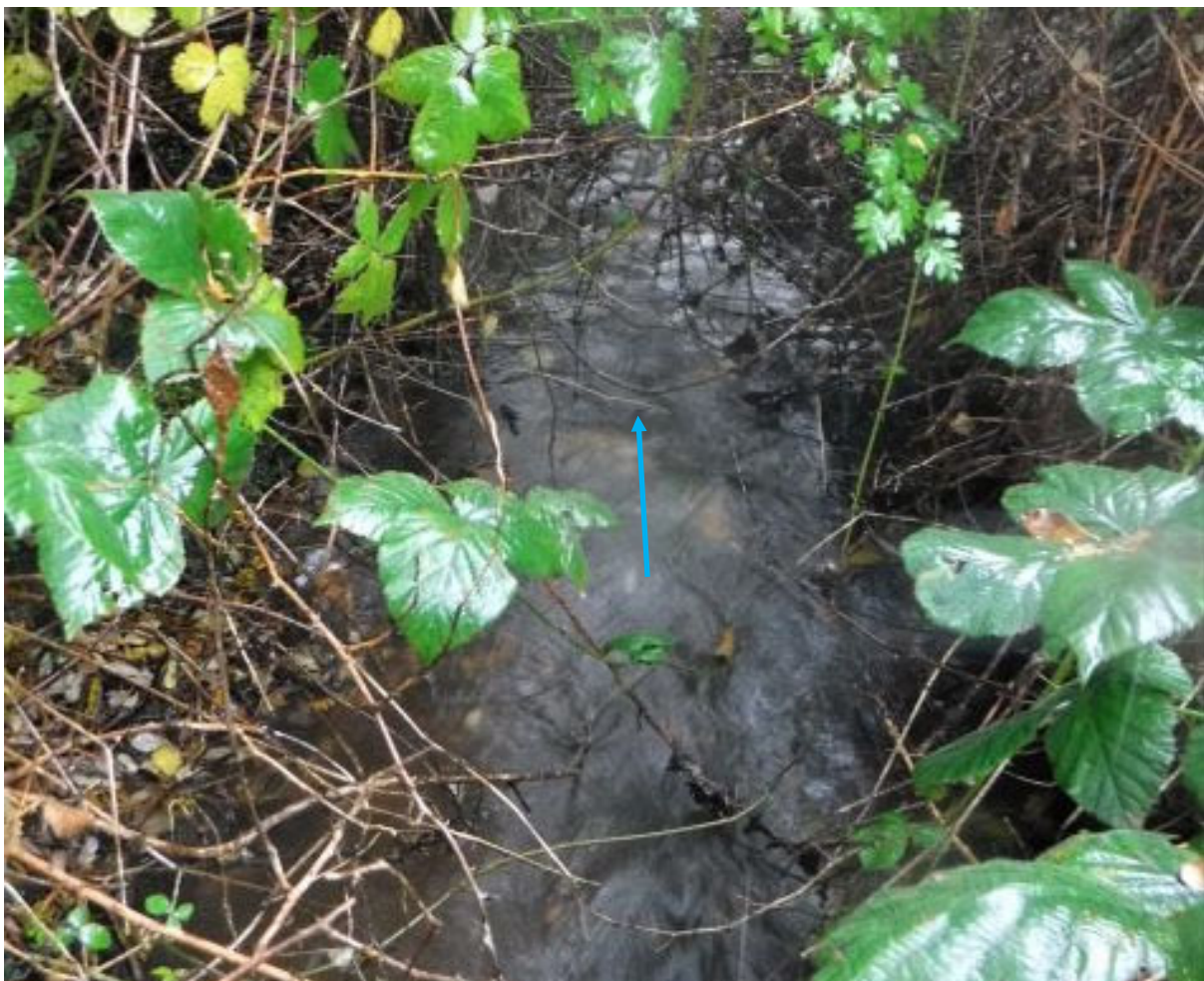
Photo 17: View of good water flow in overgrown drainage channel on east side of GAA car park.
