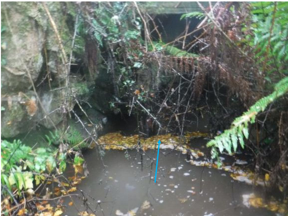
Photo 13: Start of drainage culvert from southern boundary going under St. Marys carpark area.
