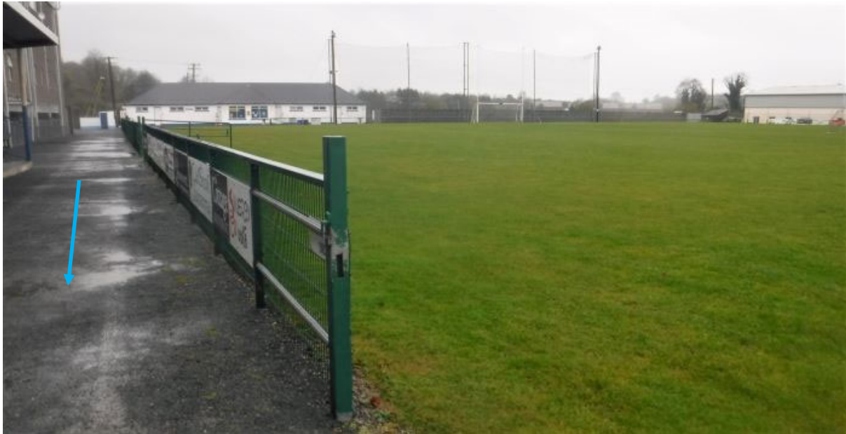
Photo 14: View North of St Marys pitch. Site drainage is culverted under path on left hand side.
