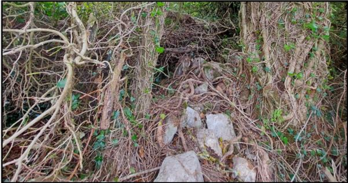
Plate 2.4 Collapsed stone wall showing densely entwined ivy vines
