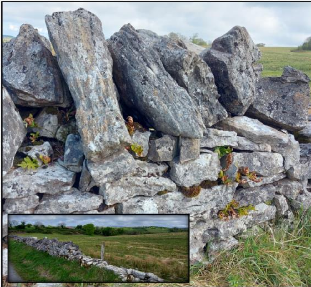
Plate 2.1 Existing stone wall habitat (BL1, Fossitt, 2000) along the southern boundary of the Proposed Development
