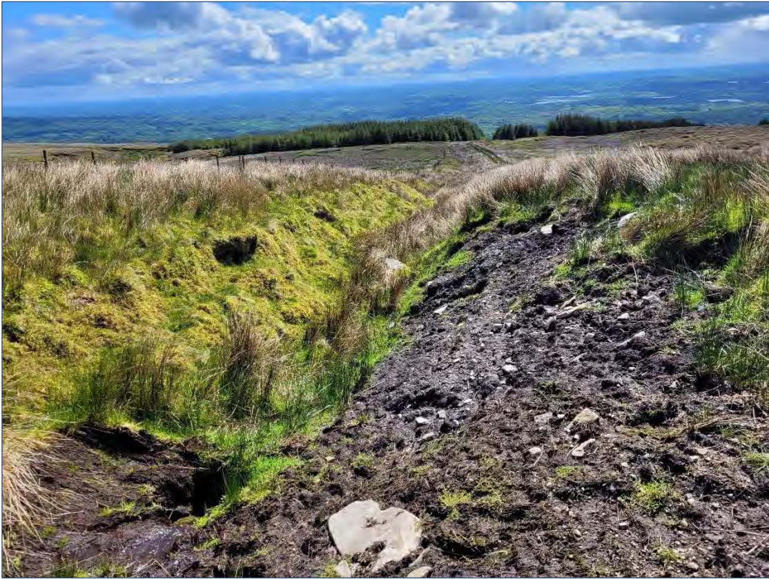
Plate 5-3 Proposed footprint for sheep's wool track over existing degraded bare soil (ED2).
