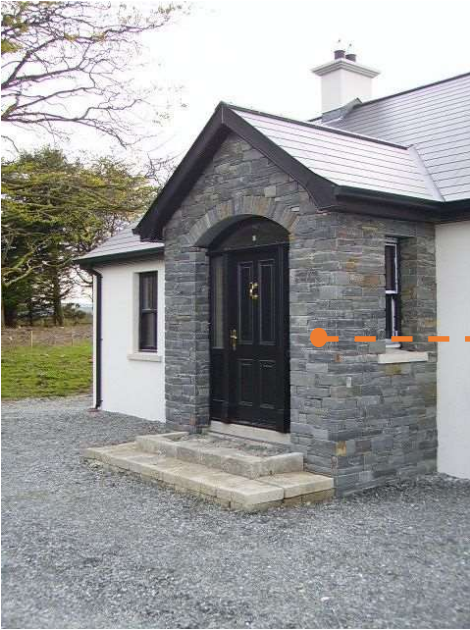
Fig 6 – Raised stone detail for selected areas on front and side elevation porches.
