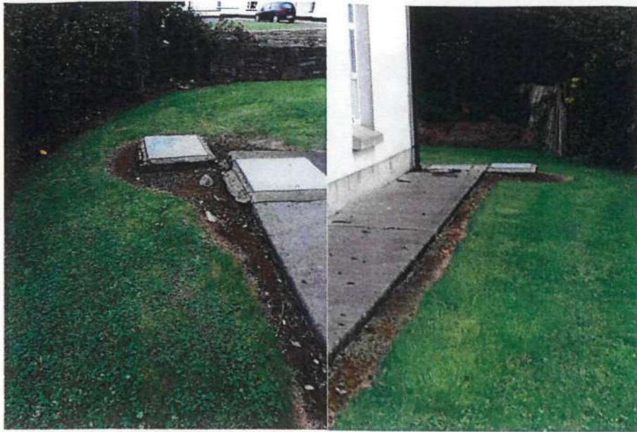
Figure 9: Chambers at rear of Mohill Health Care Centre
