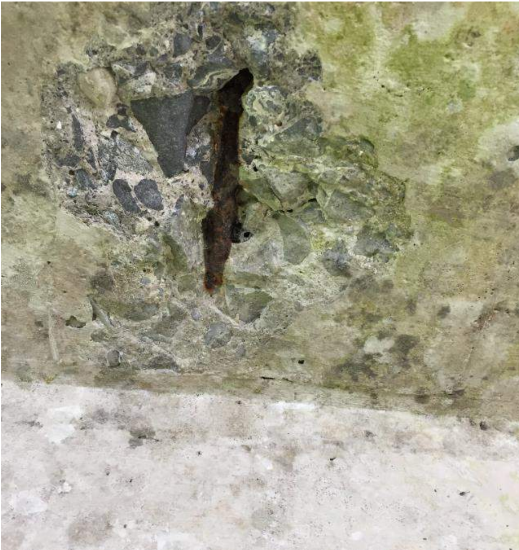
Evidence of corroded reinforcement bar in the deck slab soffit which has led to spalled concrete
