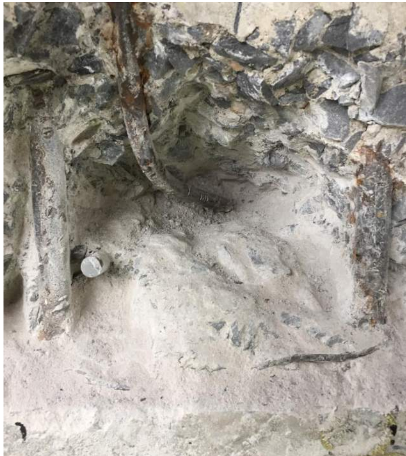
Breakout at CS3 & CB3 (column, east face – close up)
