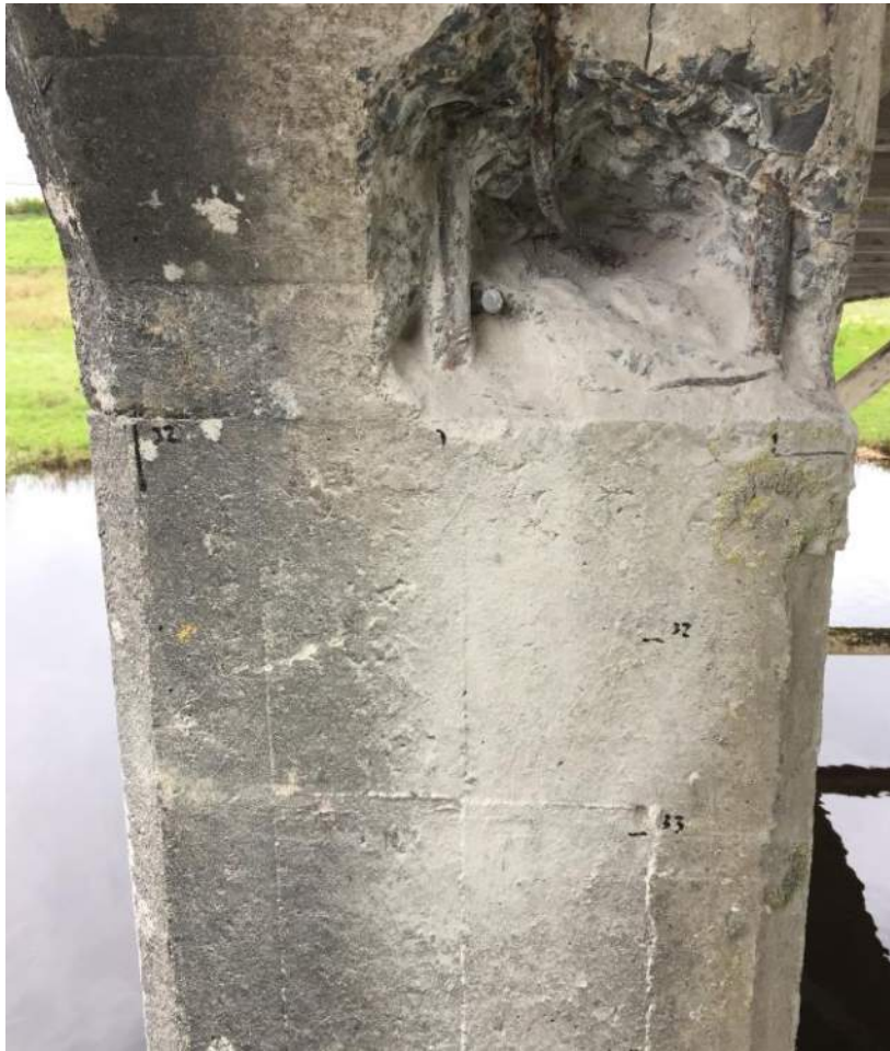
Breakout at CS3 & CB3 (column, east face)
