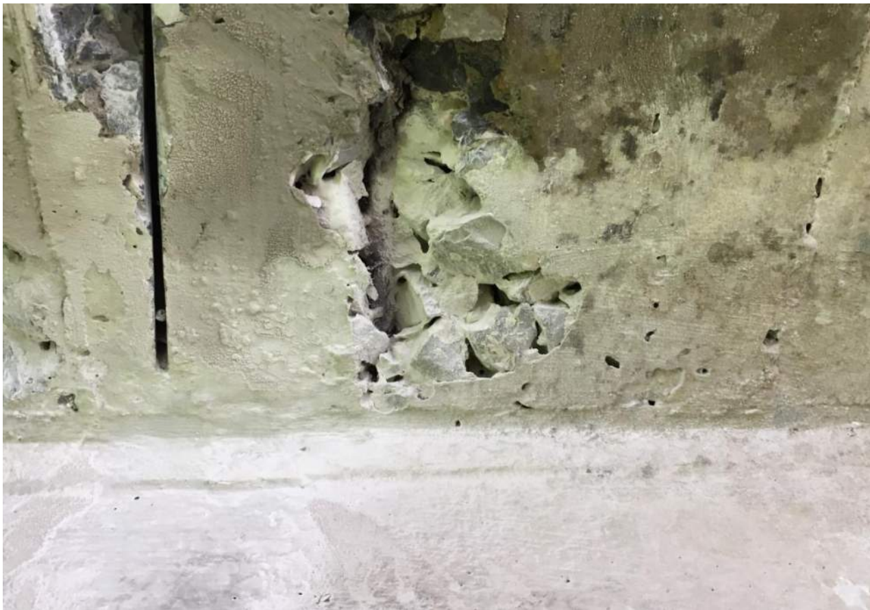
Evidence of honeycombed concrete surrounding corrode longitudinal reinforcement bar in deck
