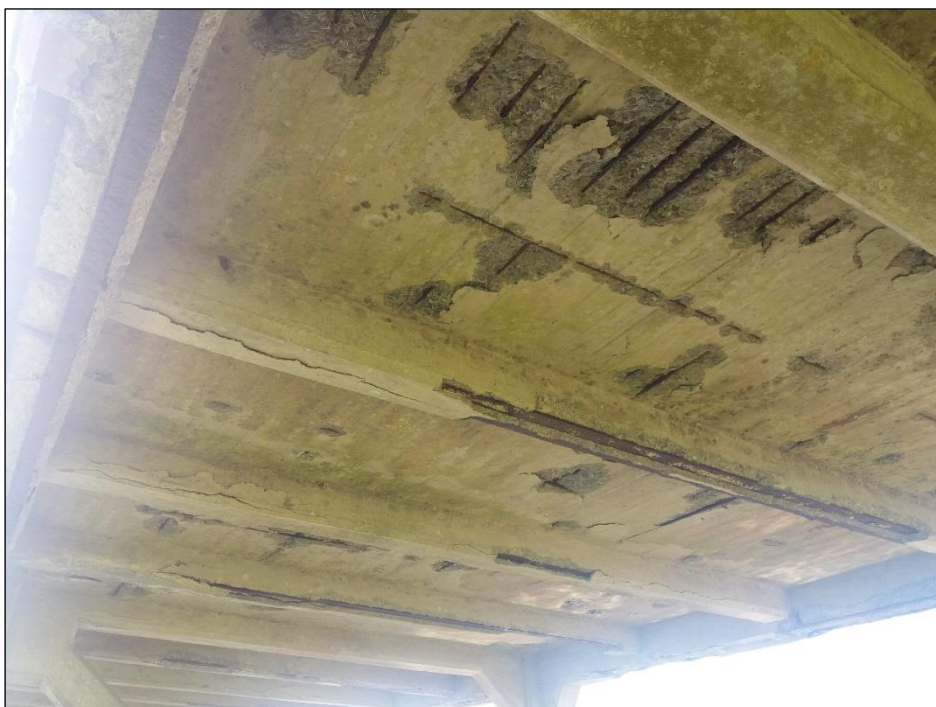
Figure 2-3: Example of extensive spalling and reinforcement corrosion
