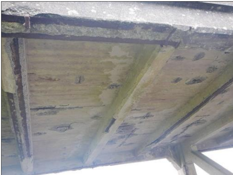
Figure 2-5: Example of extensive spalling and reinforcement corrosion
