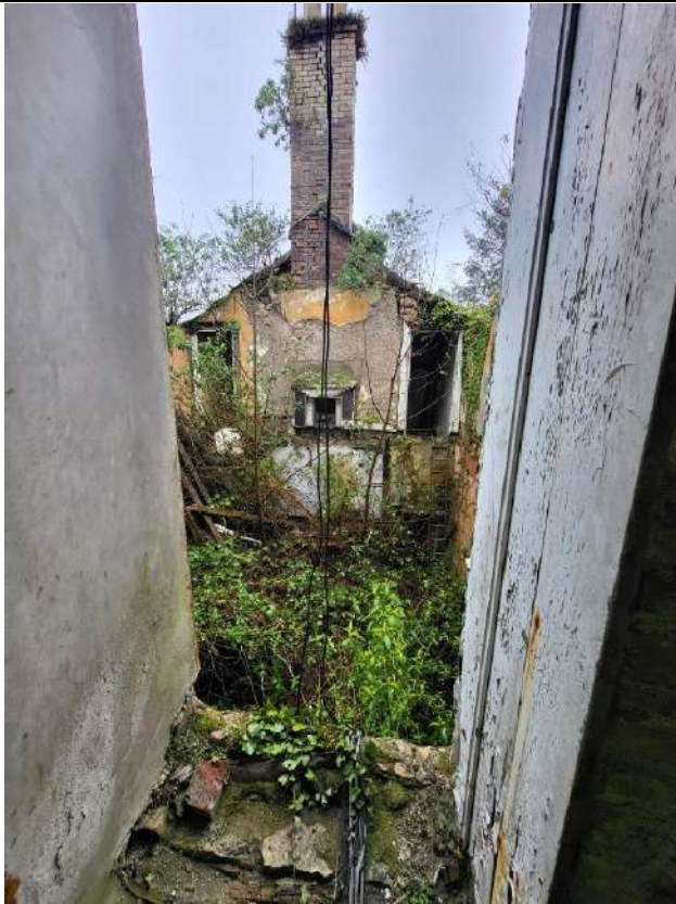
31 – View of rear (unsafe) extension
