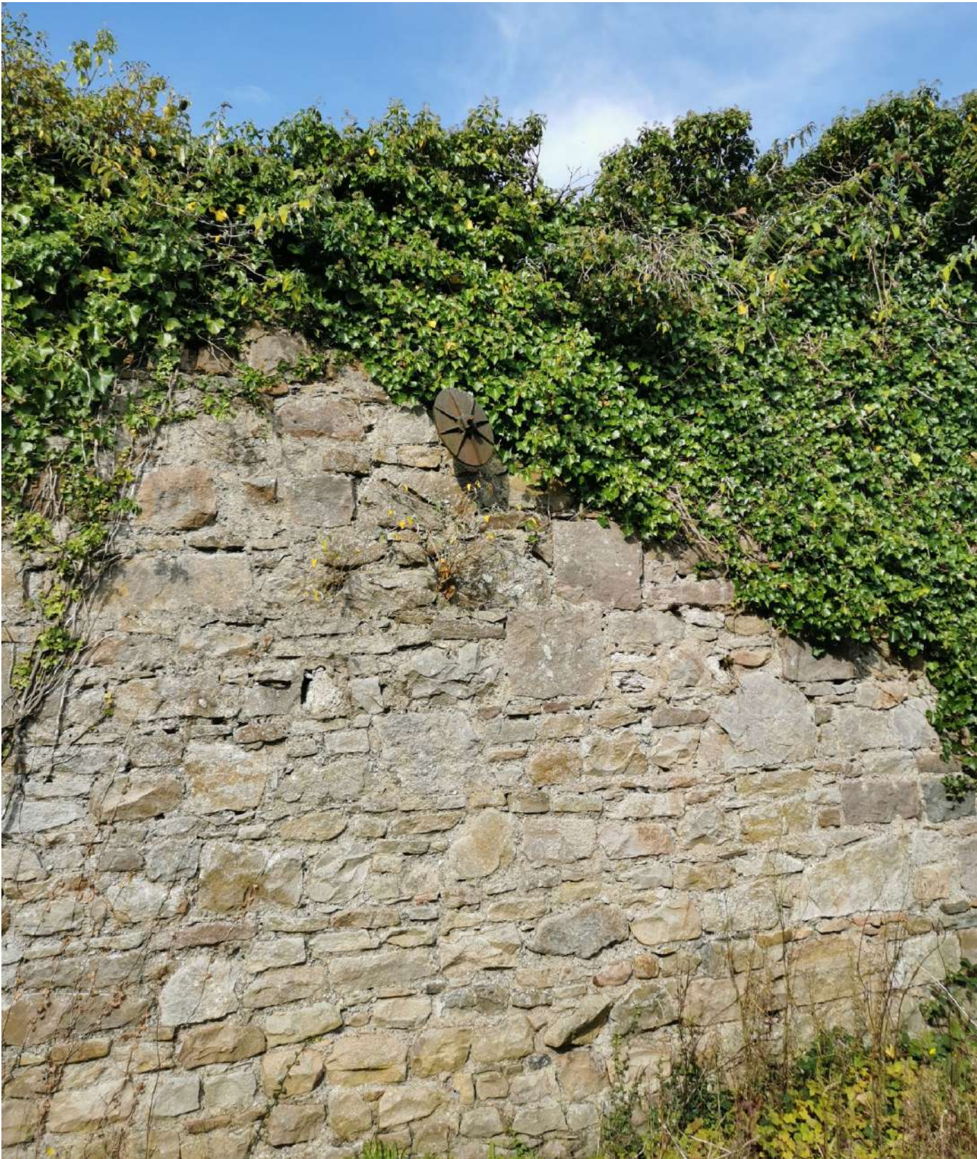
50 – Close-up view of boundary wall between the former Bank of Ireland and Market Yard carpark – taken from the former BOI side
