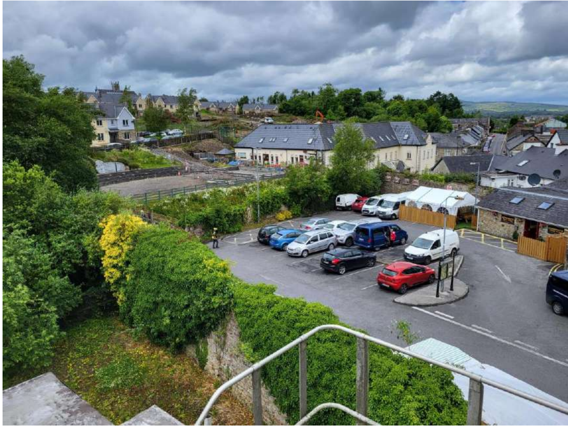
Photo 13: View of boundary wall between the car park and the rear of the former Bank of Ireland and beyond that is the boundary wall between the car park and the river.
