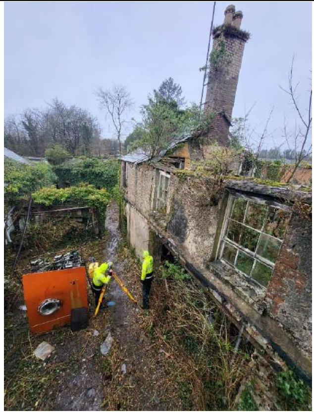
32 – View of rear (unsafe) extension
