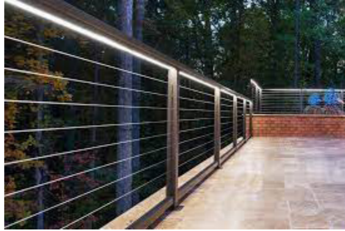
Guardrail with lighting - Installed to recess in handrail
