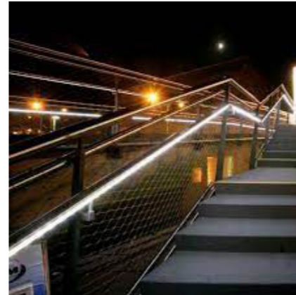
Stepped access with lighting - Installed to recess in handrail
