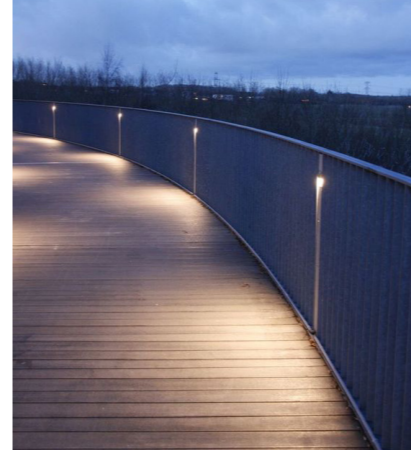
Guardrail with lighting - Installed on guardrail pillar
