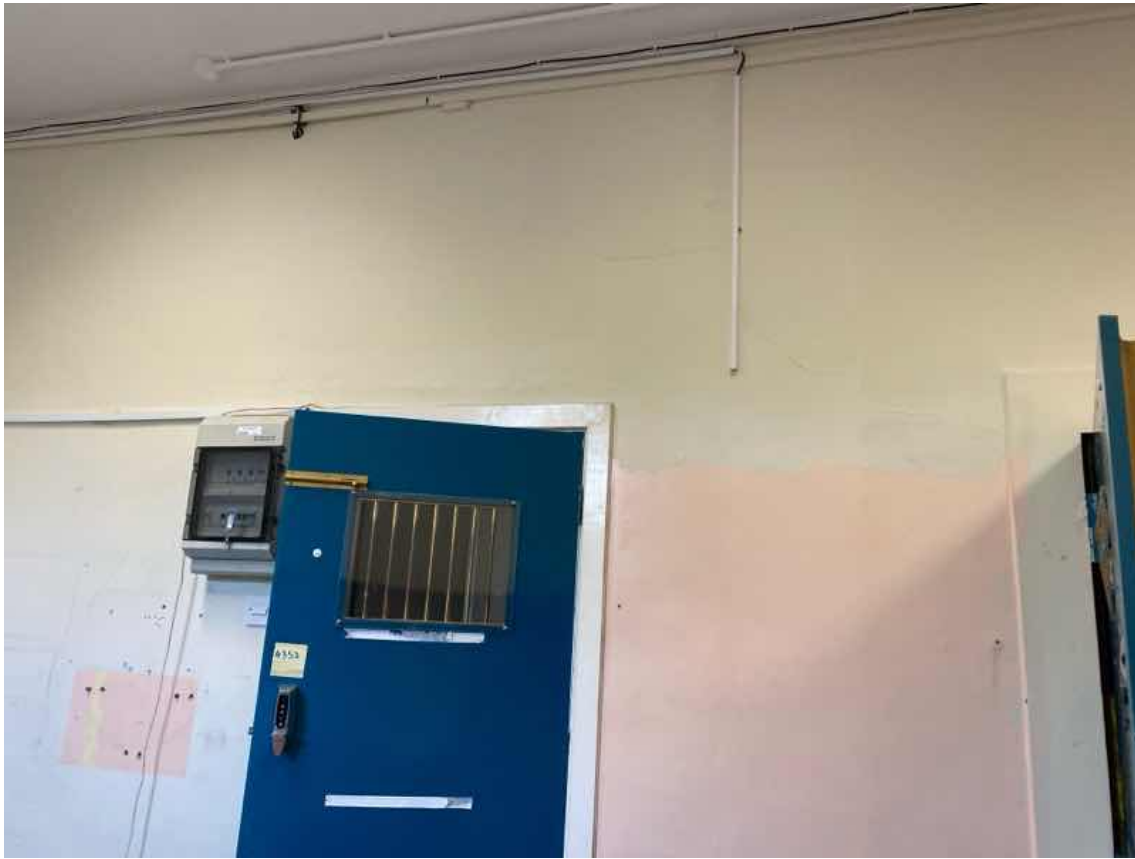
Hairline cracks on walls
