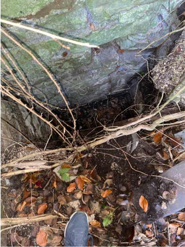
Deep pit and drainage hole in wall at back wall
