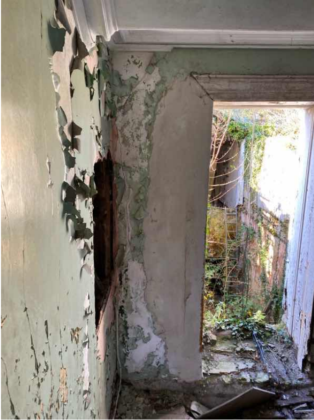
Evidence of significant damp ingress on wall adjacent to window
