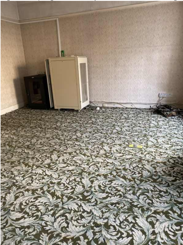
Significant spring in floor , likely as a result of under designed timber joist which span parallel to front exterior wall
