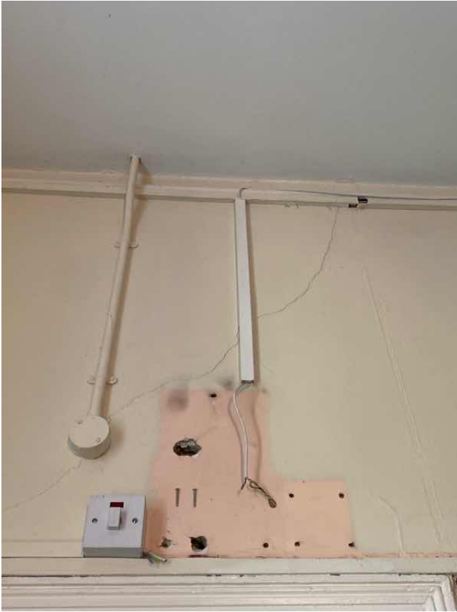
Hairline crack above door
