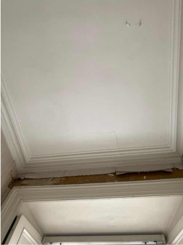
Observed hairline cracks in Cieling, generally in satisfactory condition
