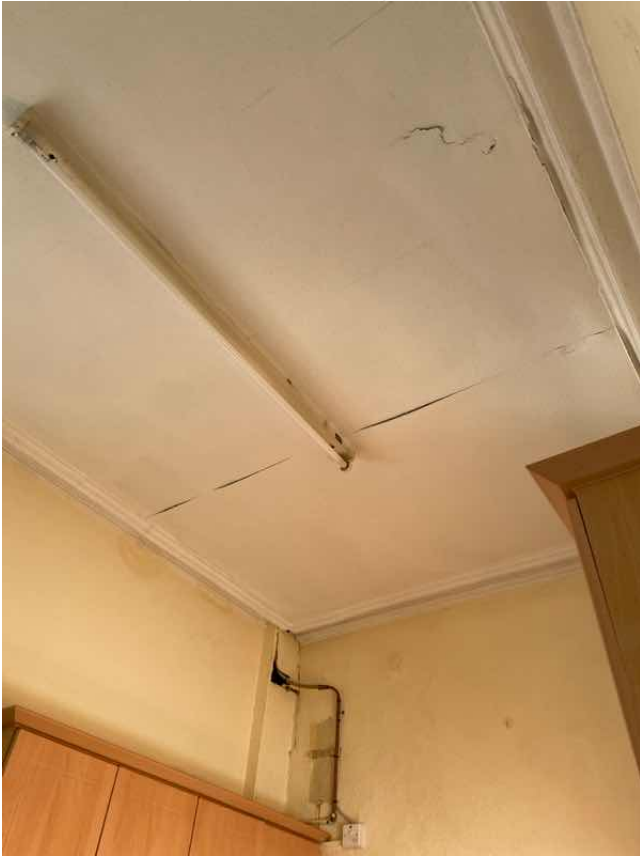
Wallpaper coming away from ceiling
