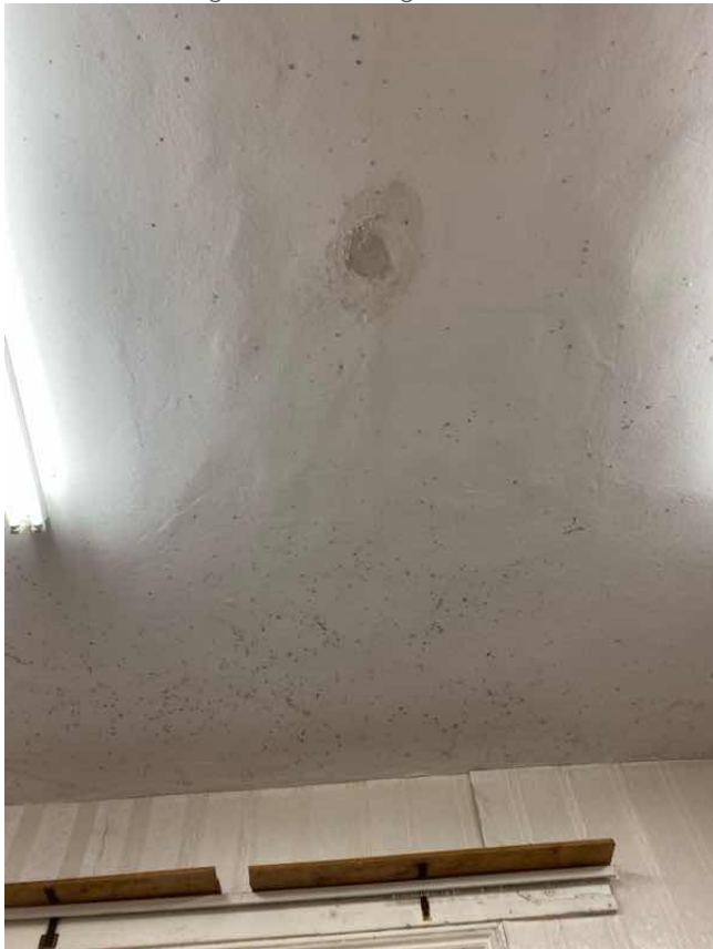
Extensive mould growth on Cieling
