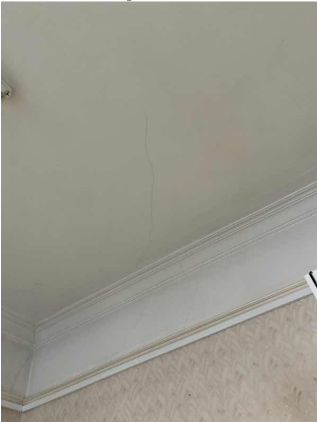
Hairline cracks in Cieling
