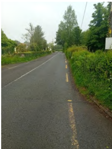
Plate 1. Looking north from junction with R281 along the R282, route for sewer pipe.
