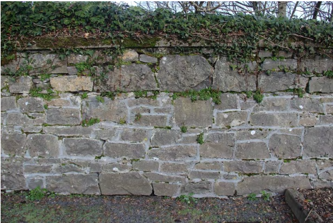
Photograph 11 - Section B Detail of Repointing with OPC
