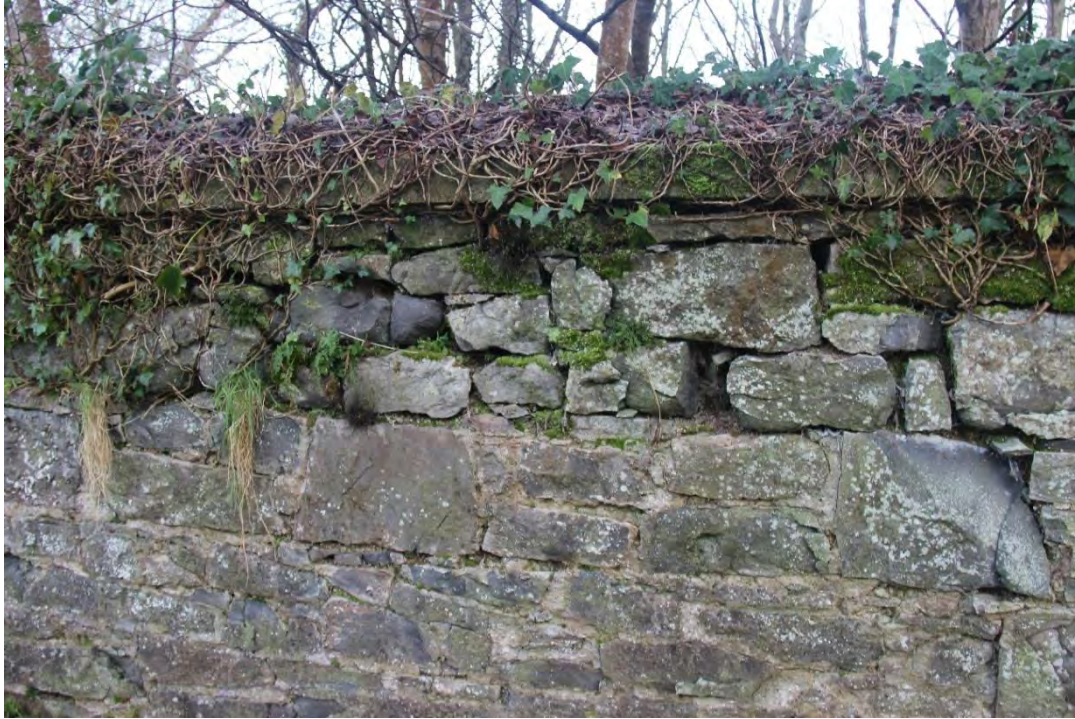
Photograph 12 - Section B1 Detail of Mortar Loss on Top level of wall
