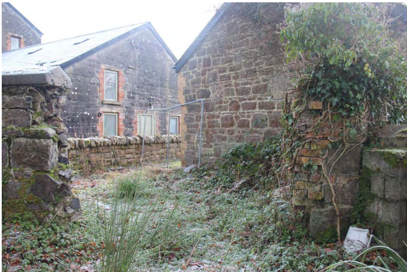
J991_P20 Existing Boundary Wall Gap in Section D
