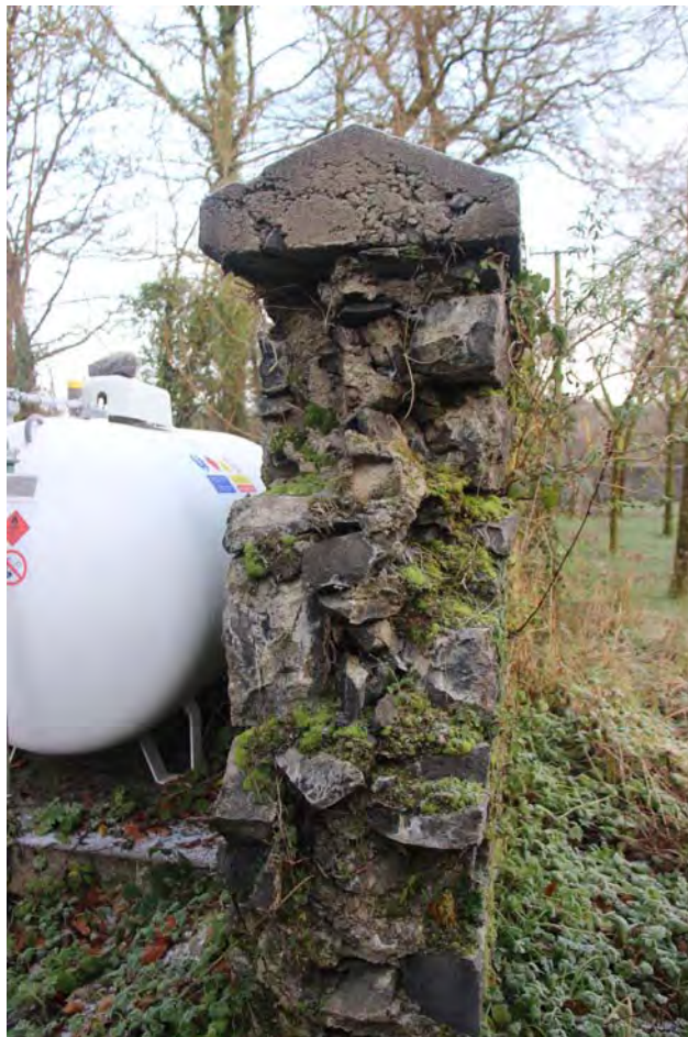
J991_P19 Existing Boundary Wall Gap in Section D
