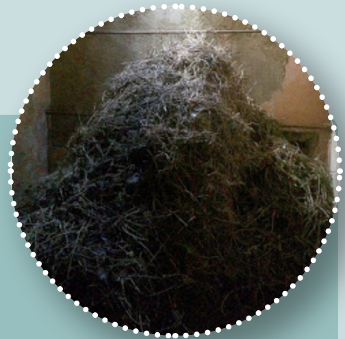
Jackdaw nest material has blocked the chimney of an abandoned farmhouse and has gathered at the fireplace
