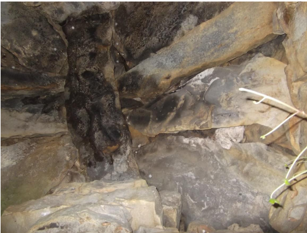
View of roof with central beam lintel and pitched side lintels (photo by D McCarthy 28 th July 2021)
