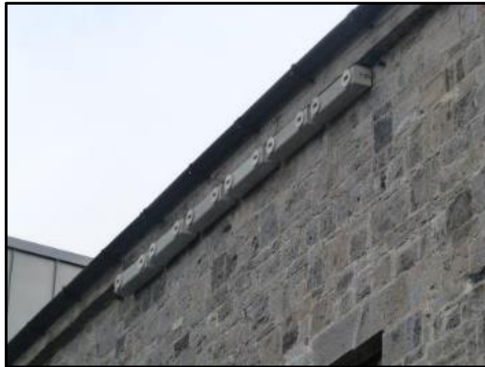
Figure 12: A row of Swift nest boxes installed at Mullingar Courthouse. Photo: Richella Duggan
