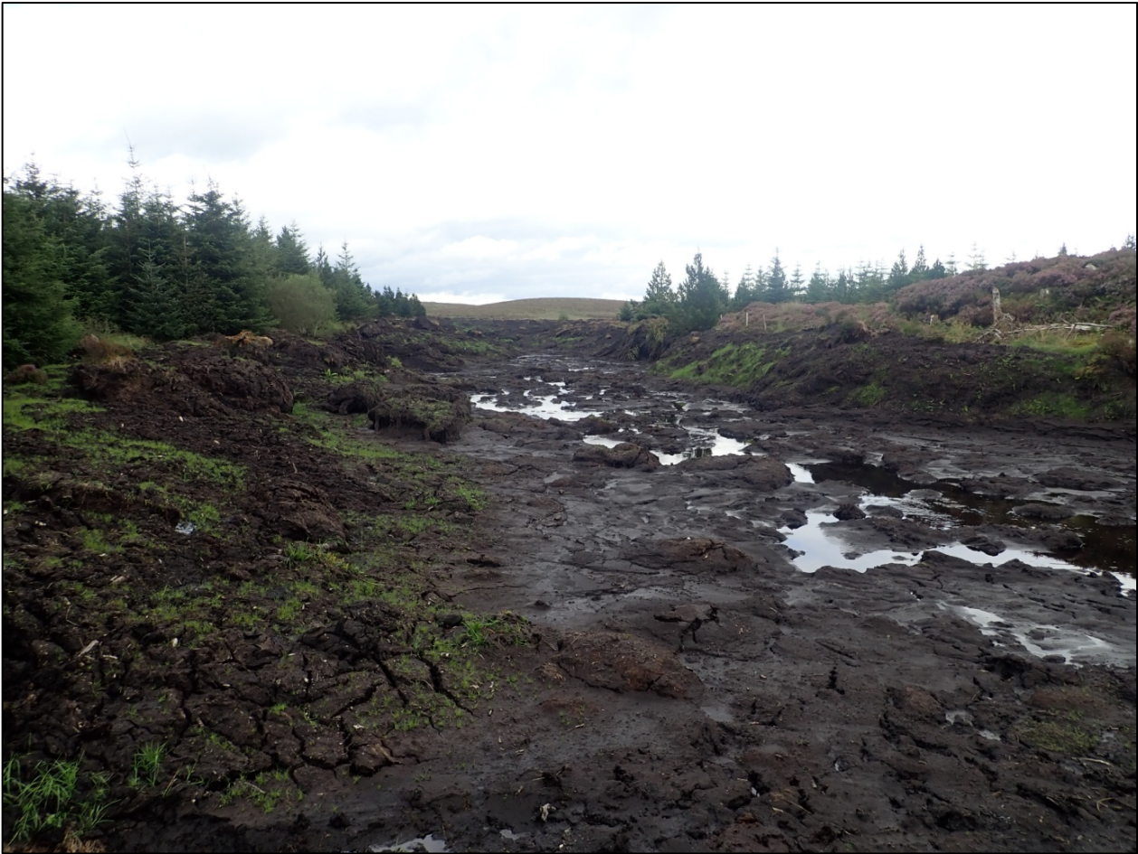
The peat slide up-gradient of the Dawn of Hope Bridge at Greaghmagh.
