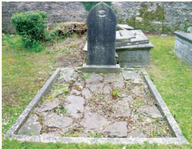
Cement deterioration is visible in this memorial surround
