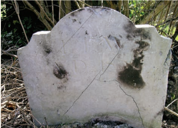
Burning in a graveyard should be avoided at all costs as it can cause severe damage to memorials
