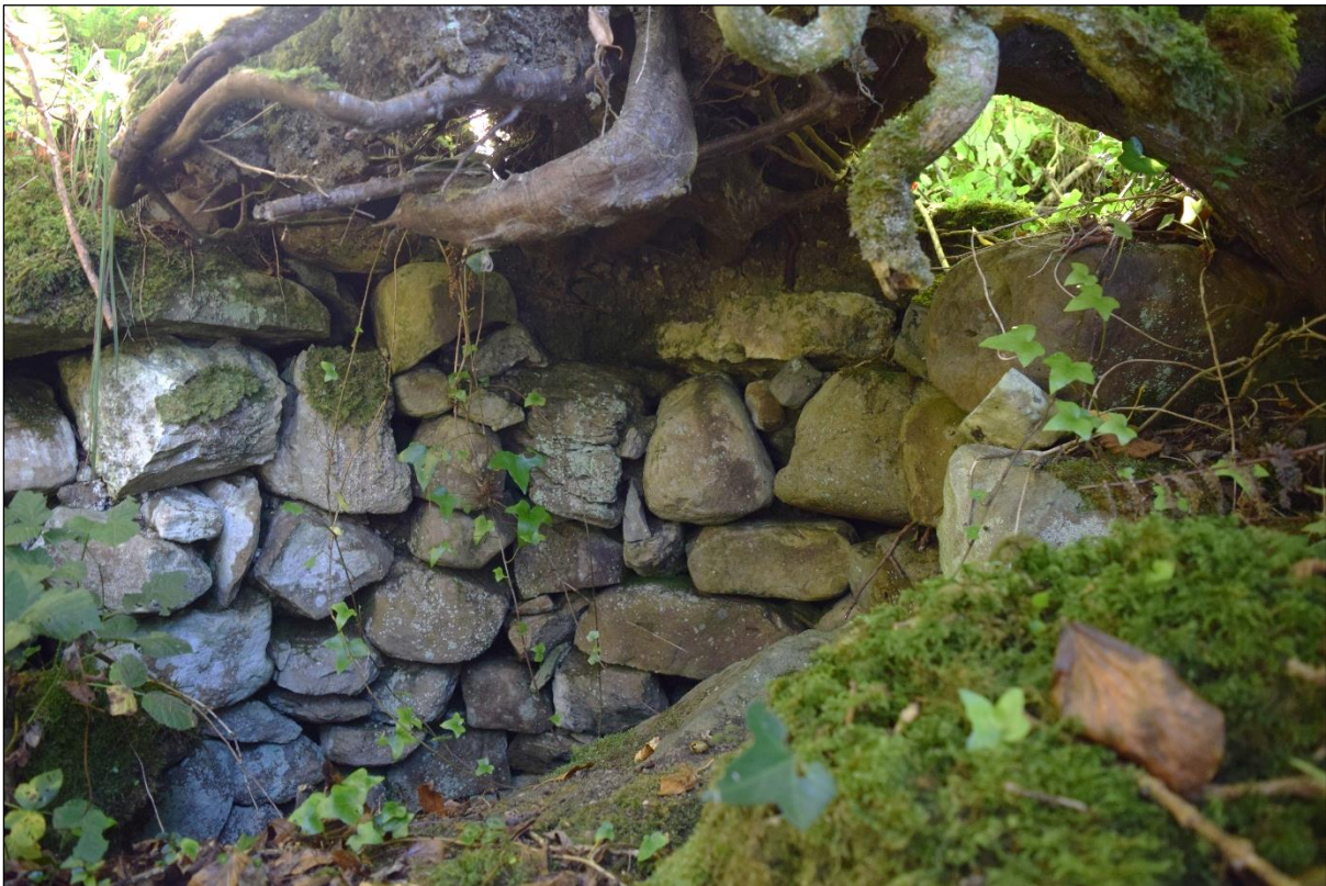
Sweathouse with collapsed roof caused by tree roots (near Rossinver)
